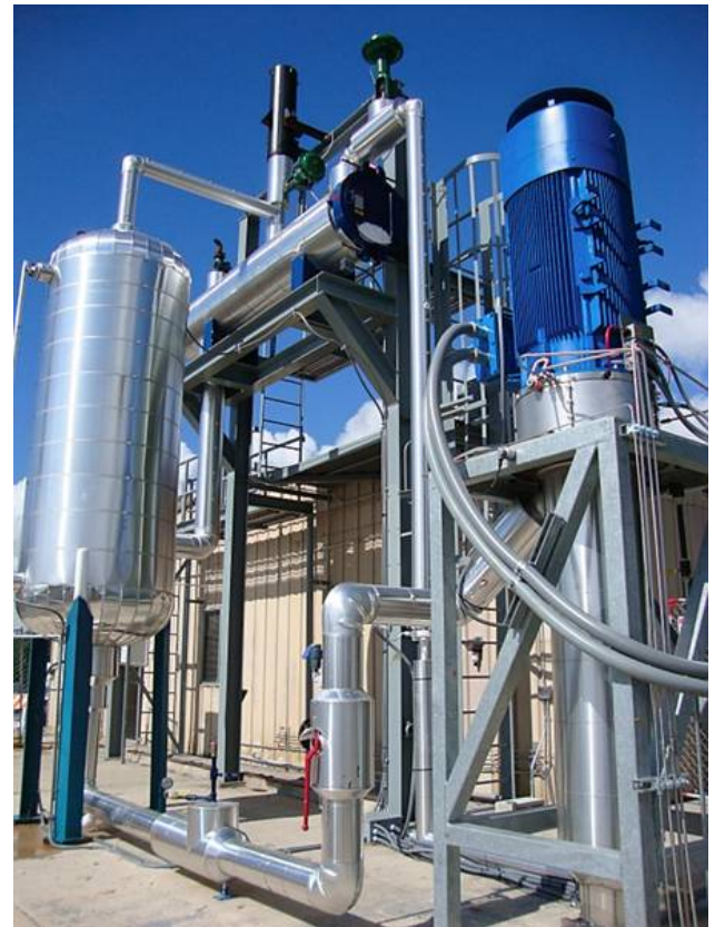
Figure 21. Photo of CO 2 Pump Test Loop
