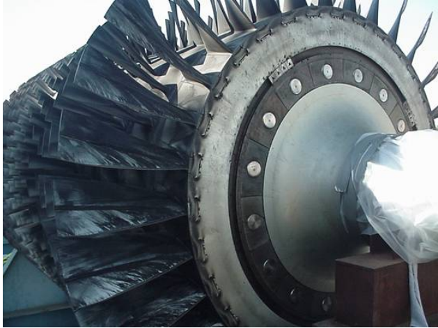
Figure 20: Oily Deposits on Axial Compressor Blades from No. 1 Bearing Oil Leakage on a Large Heavy Duty Gas Turbine
