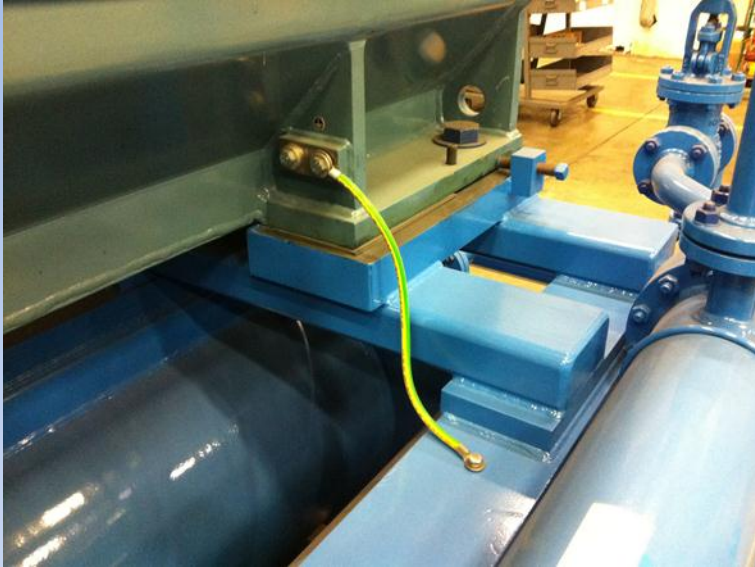
Grounding Strap on Motor.
