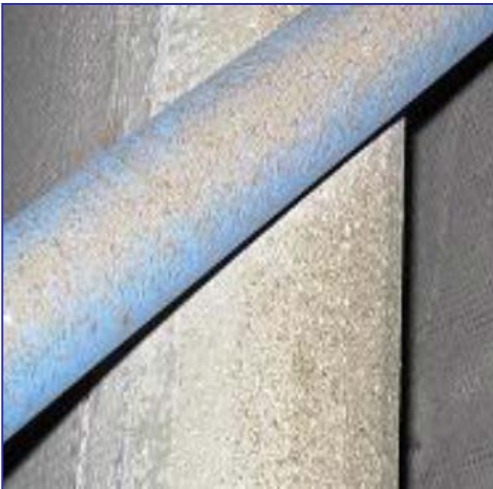
Buildup of dirt particles, chemicals, iron (rust) that eventually passed through the silencers to the compressors.
