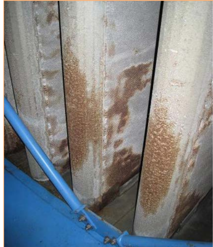
Deposits on silencers appeared to be salt, iron and dirt, all contributors to compressor fouling.
