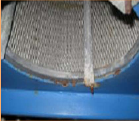
Clean side of filter contained corrosion and dirt particles.
