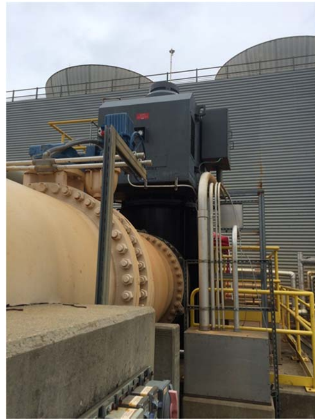
View In-Line With Discharge
