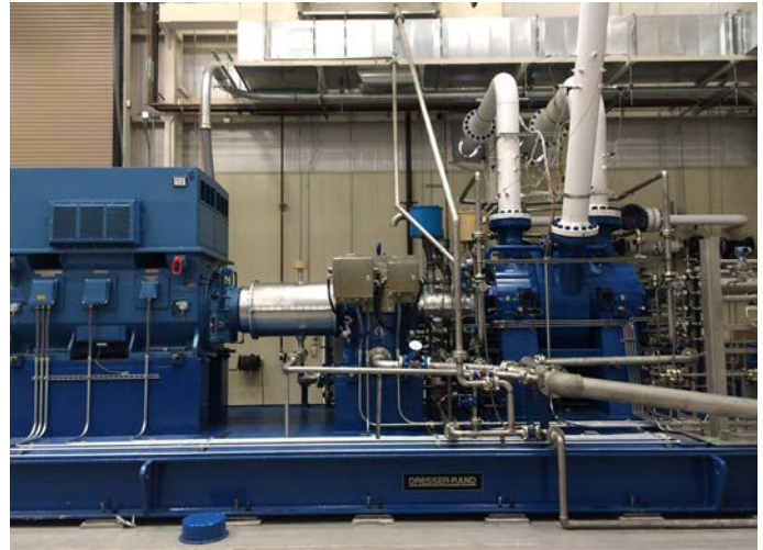
Figure 3. Installed Dresser-Rand DATUM® Compressor Package
