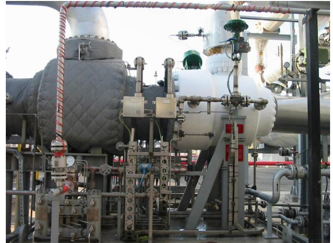
Figure 2 Operational AMB Expander-Compressor Note the diffuser cone (far –right), and white ice-ball surrounding the cold expander volute (right), and the thermal protective blanket around the hot compressor volute (left). Photo courtesy the Atlas-Copco Mafi-Trench Corporation.
