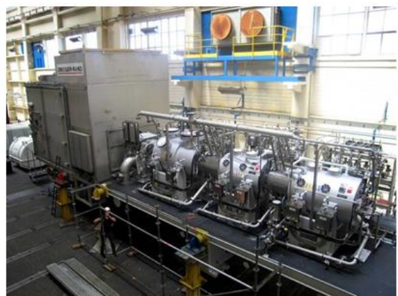
Figure 5. A three case gas reinjection compressor train driven by an aero-derivation gas turbine destined for installation on an FPSO.
