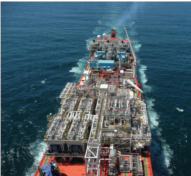
Figure 6. Two 27 MW steam turbine generator sets on board the Knock Allan FPSO for power generation.
