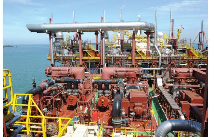
Figure 7. Three 24 MW condensing steam turbine generator sets on board the Peregrino FPSO.
