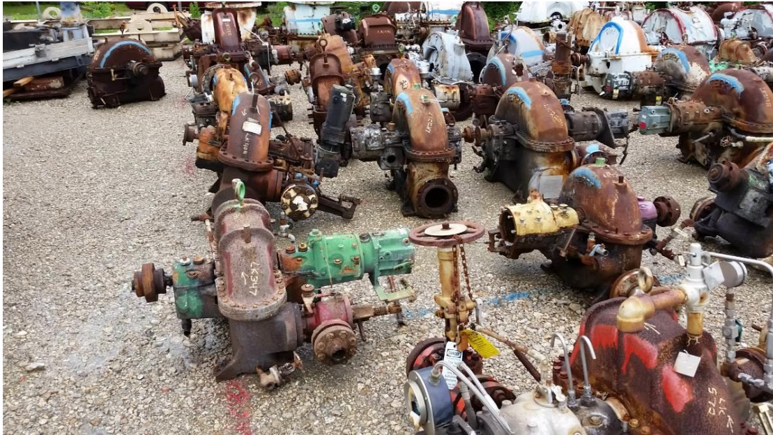
Figure 4: Surplus turbines at Keene Turbomachinery Services.
