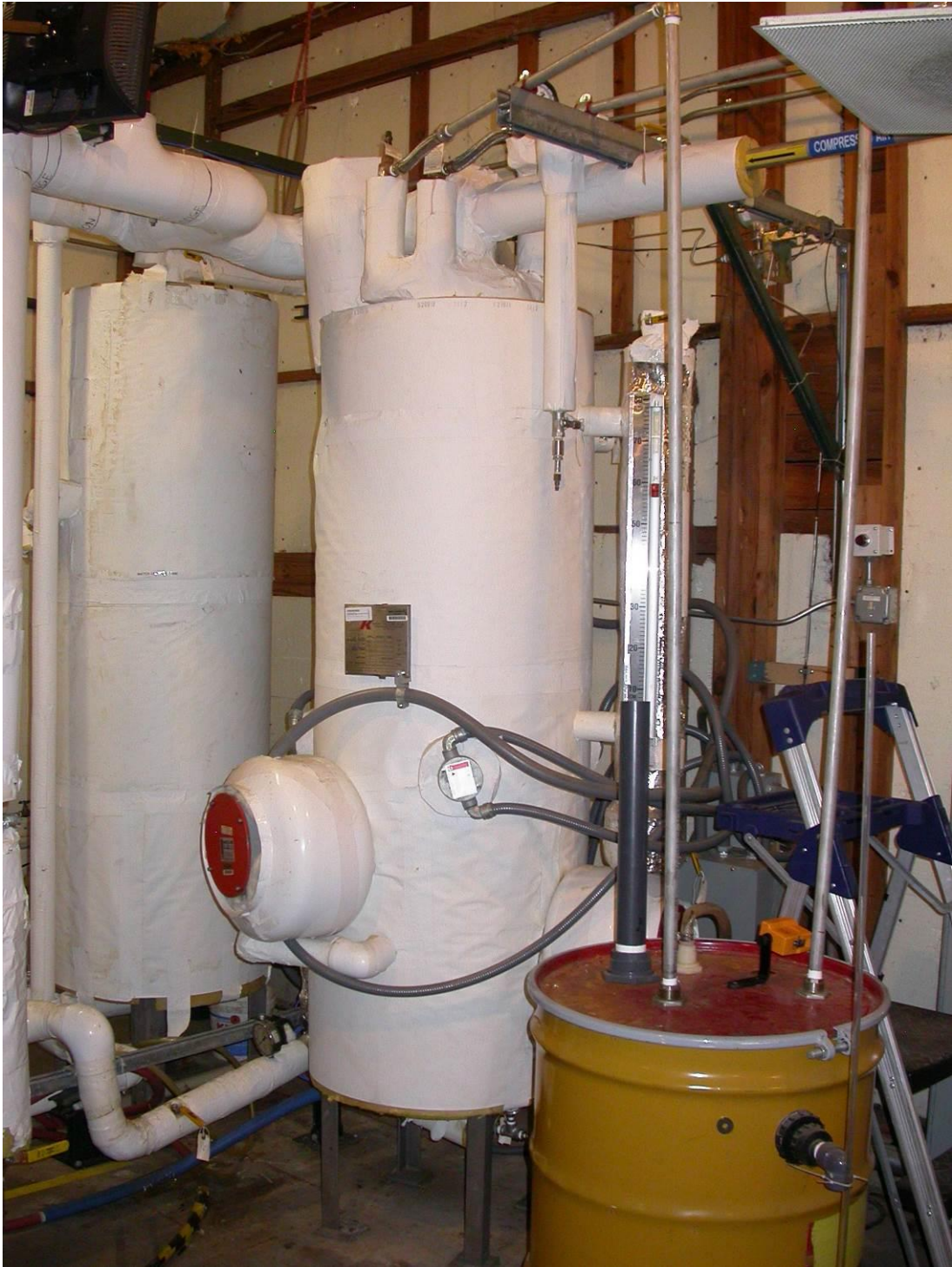
Figure 16: Steam generator and blowdown drum.
