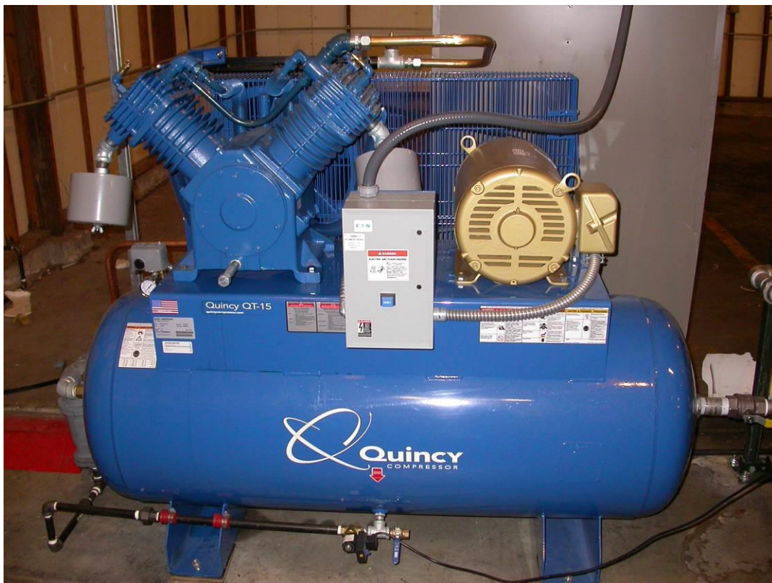
Figure 18: Facility air compressor.
