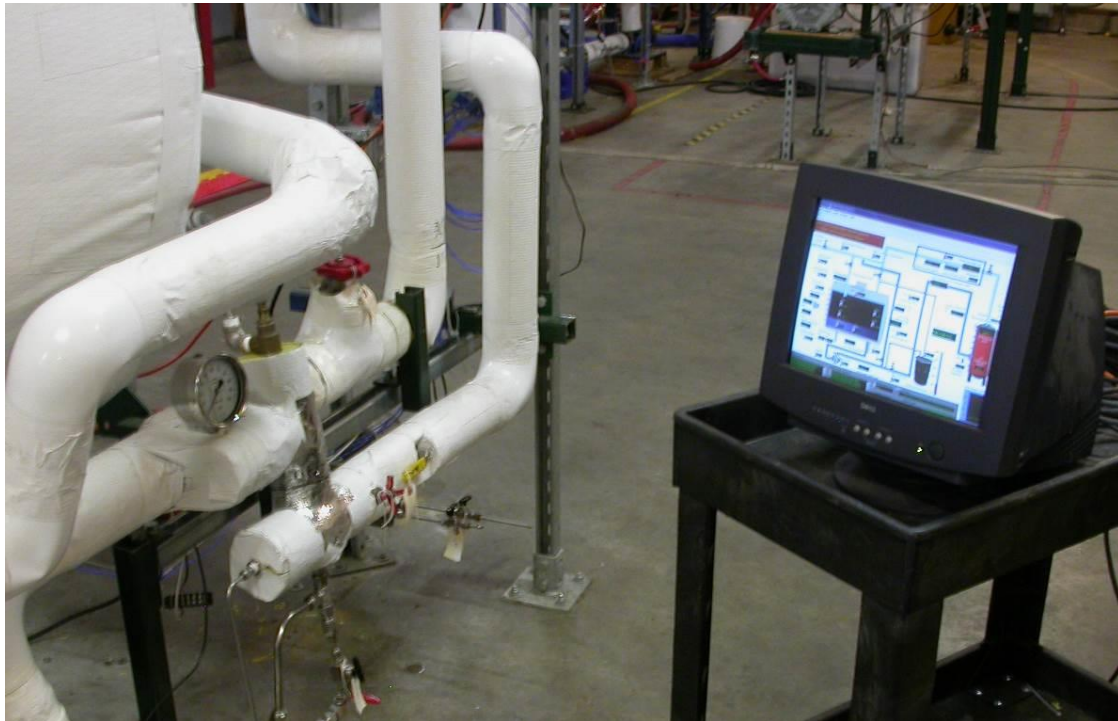
Figure 21: Water injection control station.
