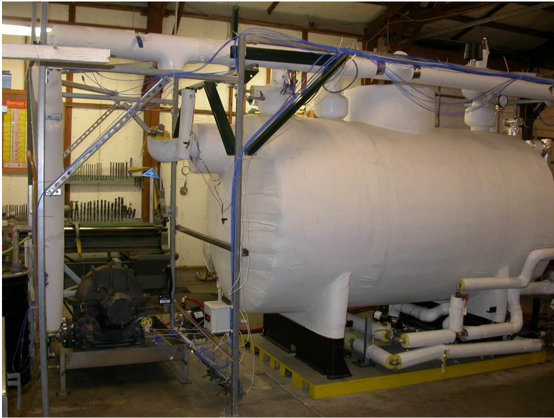
Figure 17: Feedwater storage tank and turbine.
