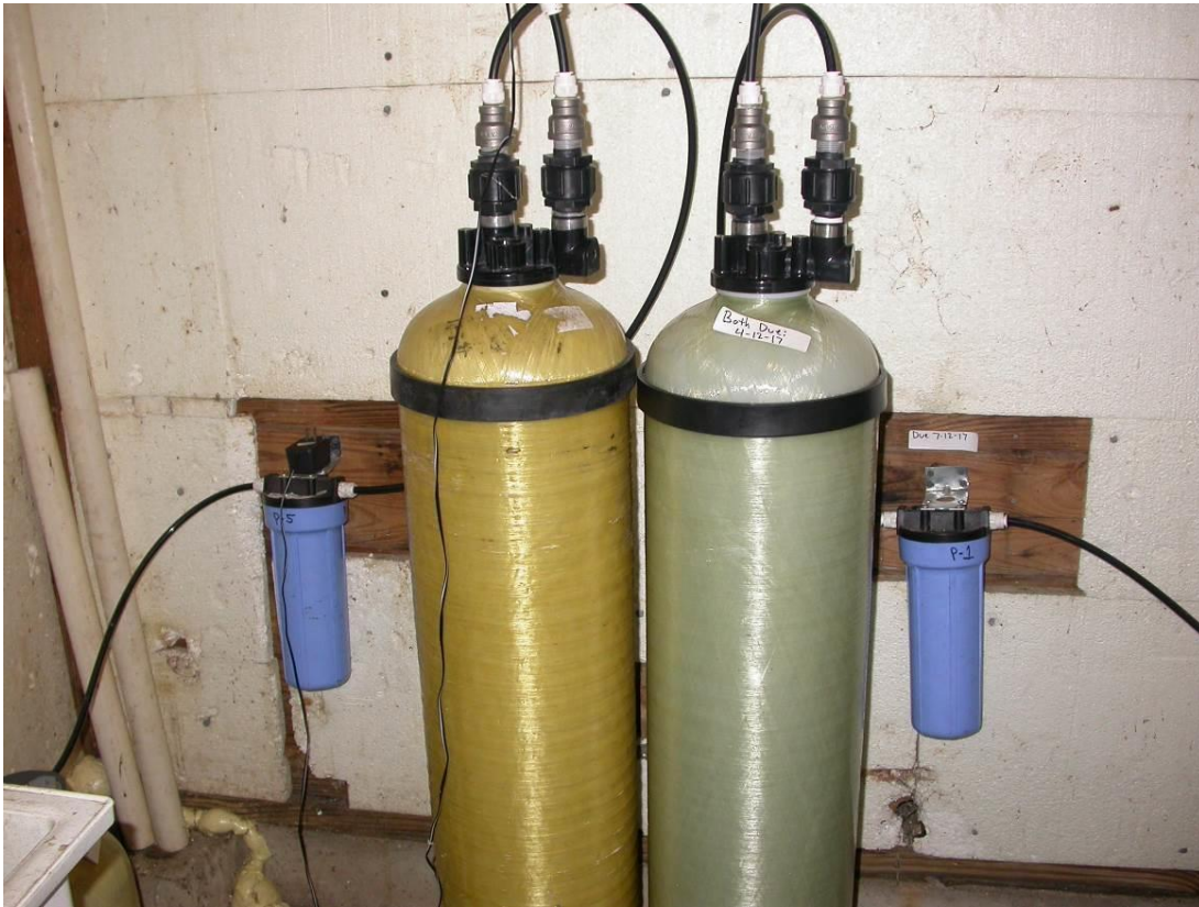
Figure 15: Cartridge filter and resin tanks for deionization system.
