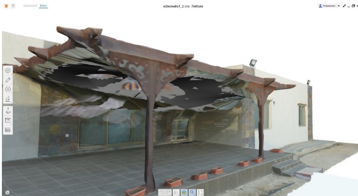
Figure 7. Distorted mesh beneath the overhang.
