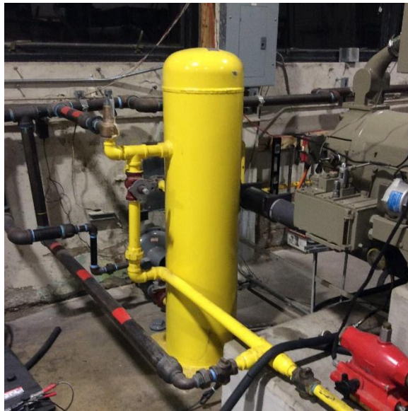
Figure 2-6: Surge tank installed in gas line
