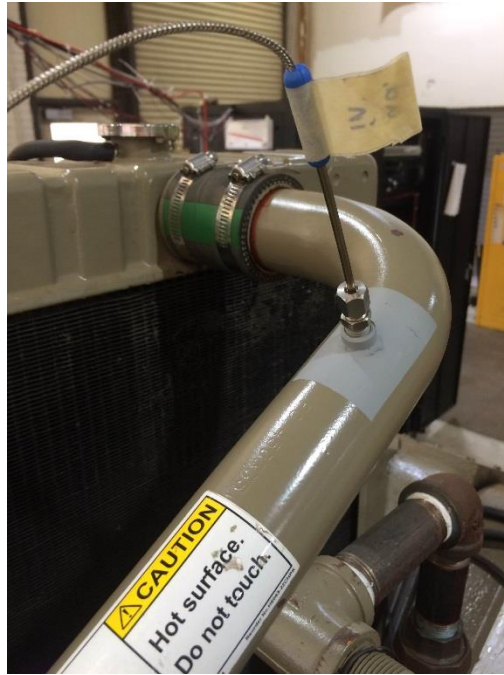
Figure 2-4: Thermocouple mounted before radiator
