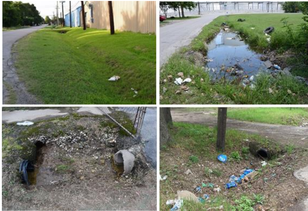
Figure 3.5. Examples of Open Ditches at Various Condition Levels
