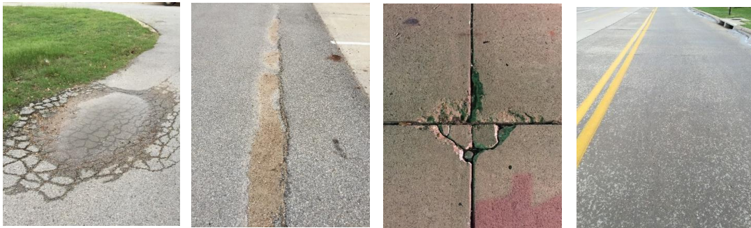
Figure 4.1. Types of Pavement Distresses (Left to Right: Depression and Block Cracking, Lane Shoulder Drop-Off, Corner Break, Polished Aggregate)
