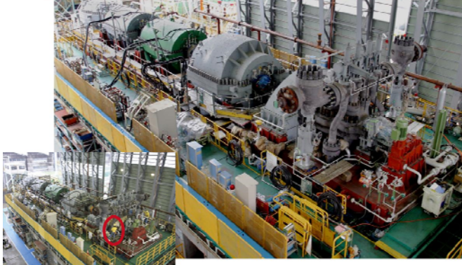
Figure.4 Recent Steam Turbine Range for Mega Crackers - Simple Single Train Solution
