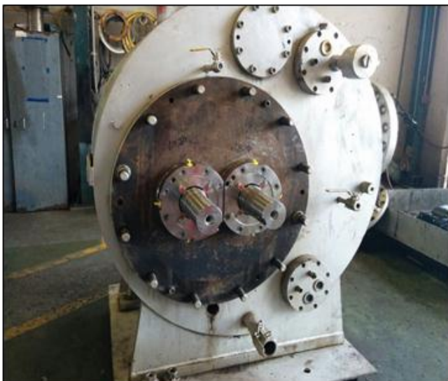
Figure 1: The Twin-Screw Pump layout with the installed mechanical seals
