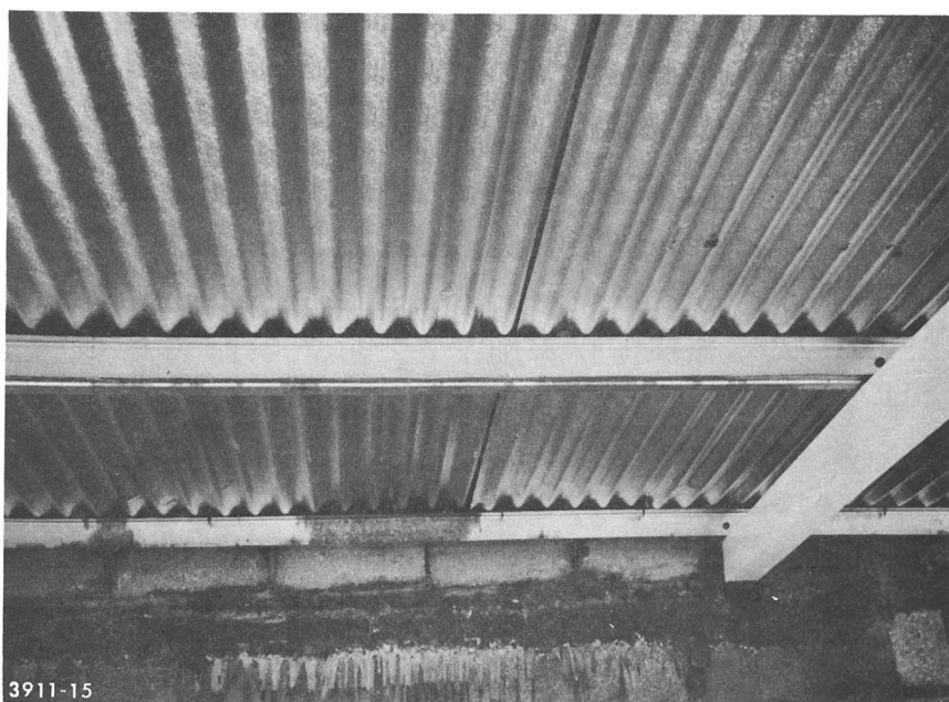
(b) Steel I-beams at World Bank Site and Service project, Spanish Town, Jamaica
