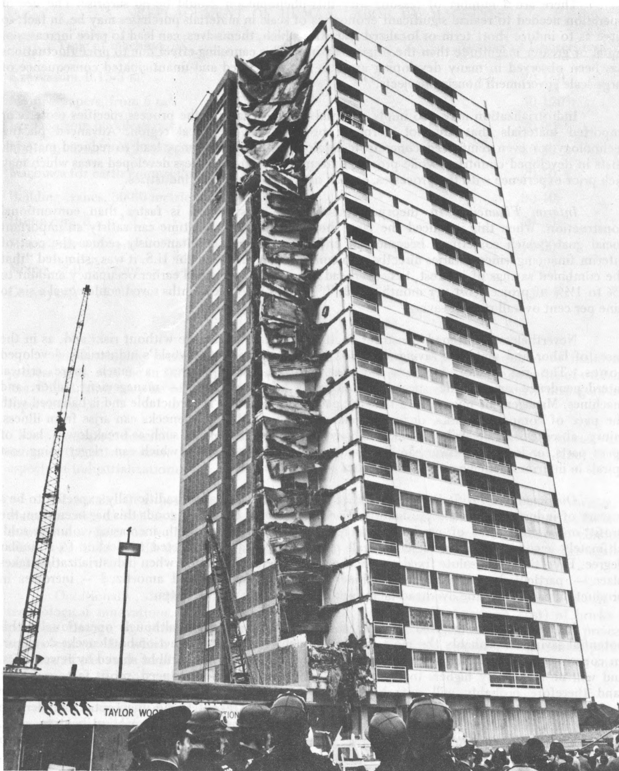
MASS-PRODUCED ERROR — An inherent danger of high-speed mass production techniques is that a single error may be rapidly proliferated. Such an error led to this fatal structural collapse in an industrialized building at Ronan Point, England, in 1969.
