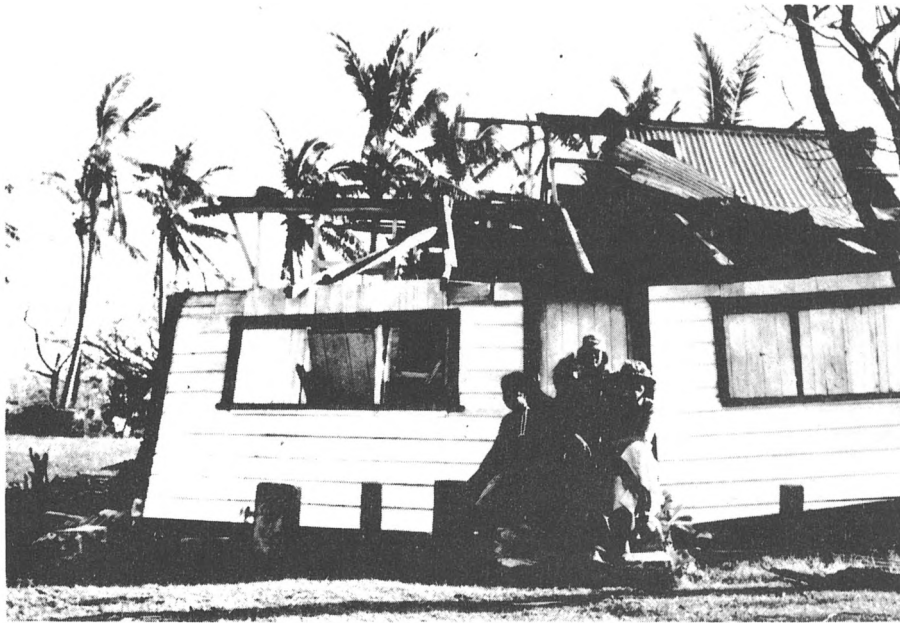
Inadequate connections between roof and walls; Inadequate connections between walls and foundation posts.
