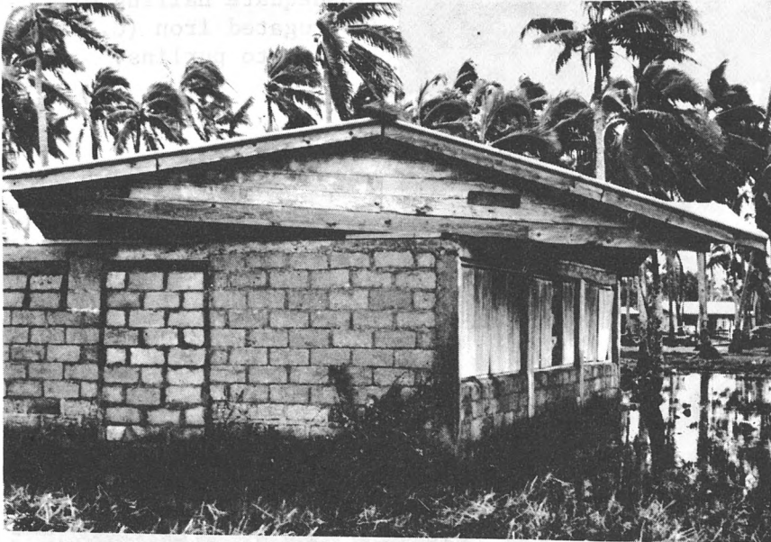
Inadequate connections between roof and walls.
