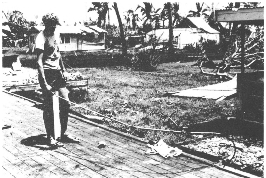
This man is holding a hurricane strap that was connected up to the wall plate. Obviously there were not enough straps used.
