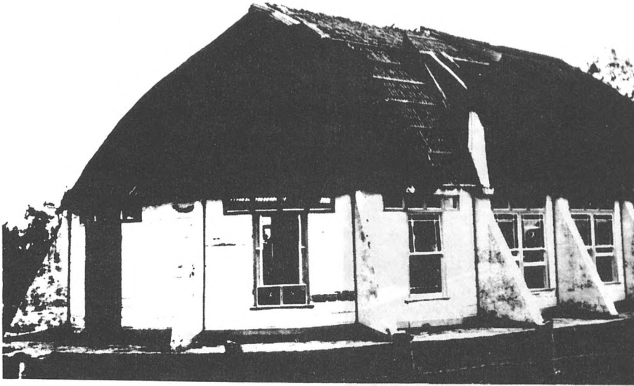
Inadequate nailing of corrugated iron (C.I.) sheets to purlins.
