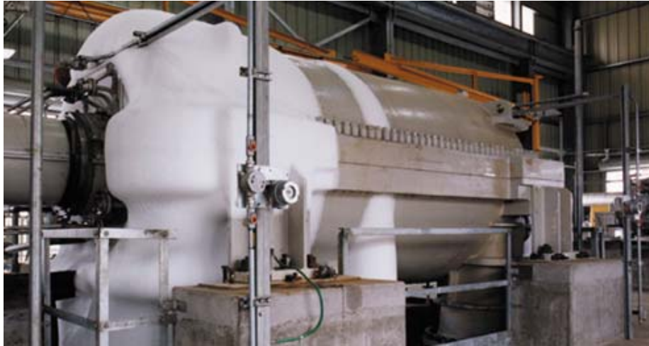
Figure 10: A centrifugal compressor with an intermediate connection in refrigeration service
