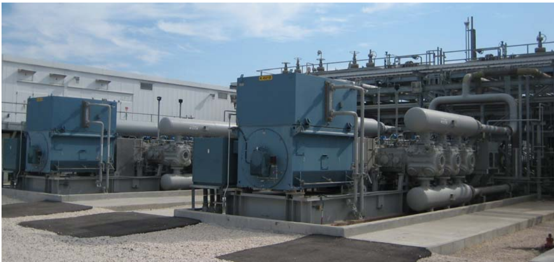
Figure 9: Motor-driven reciprocating compressor units in hydrogen service
