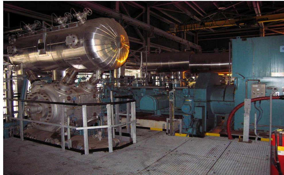
New compressor at commissioning
