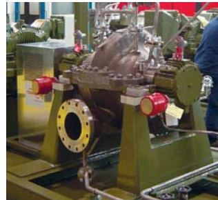
Figure 10: “Near-centerline” mounted BB1
