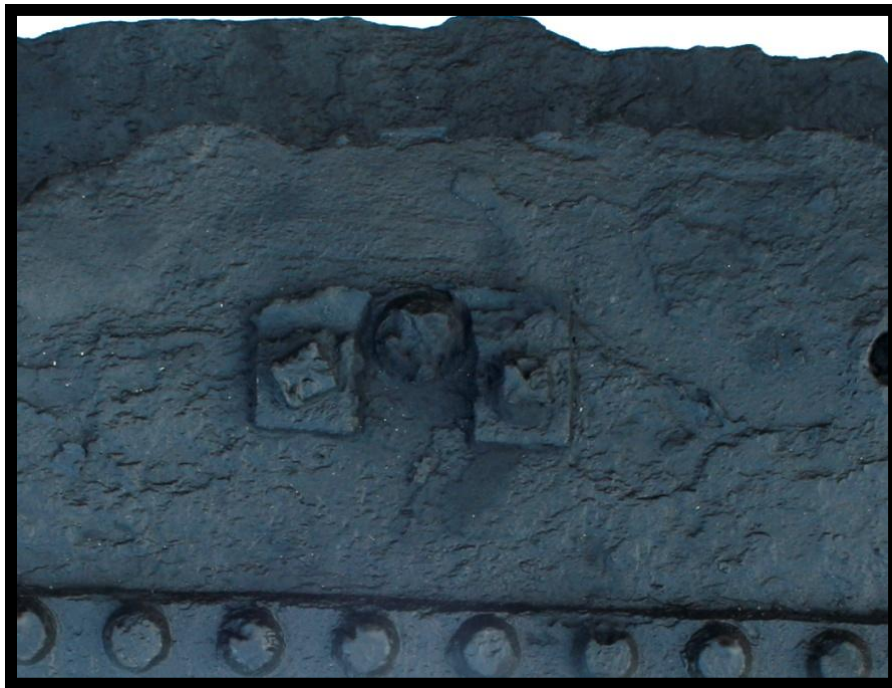
Figure 134. Broken tab for supporting bearing bars (close up shot from water leg; Artifact 132-001.79; also seen in Figure 120).
