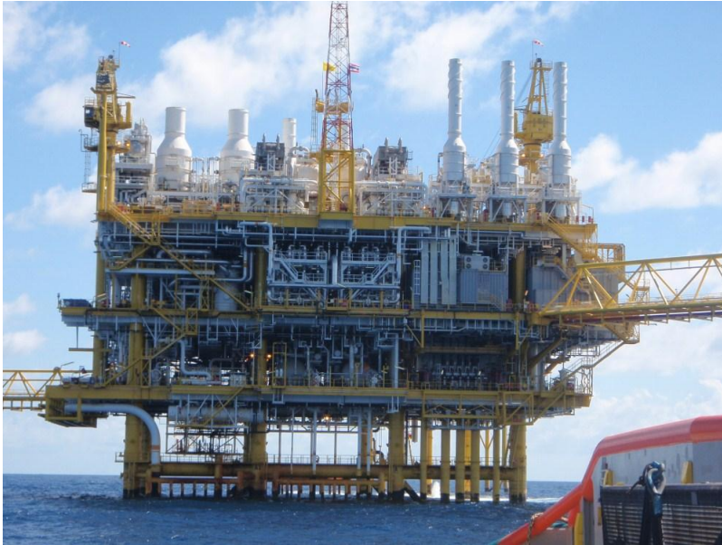
Figure 2: An Example Offshore Production Facility ("Offshore Production Platform," 2011)
