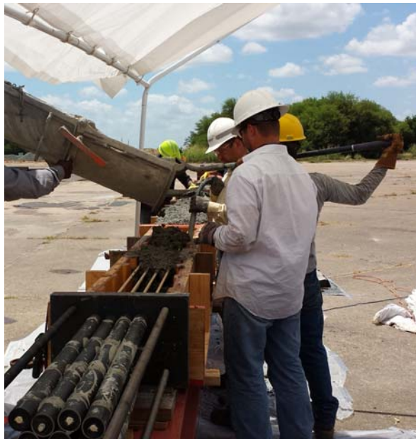
Figure 35: Pouring the concrete into the molds and using light vibration to help flow of concrete
