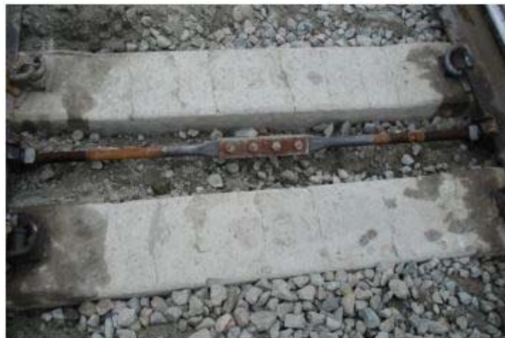
Figure 2: Cracked concrete rail ties with gauge holding bar installed post-accident (NTSB)
