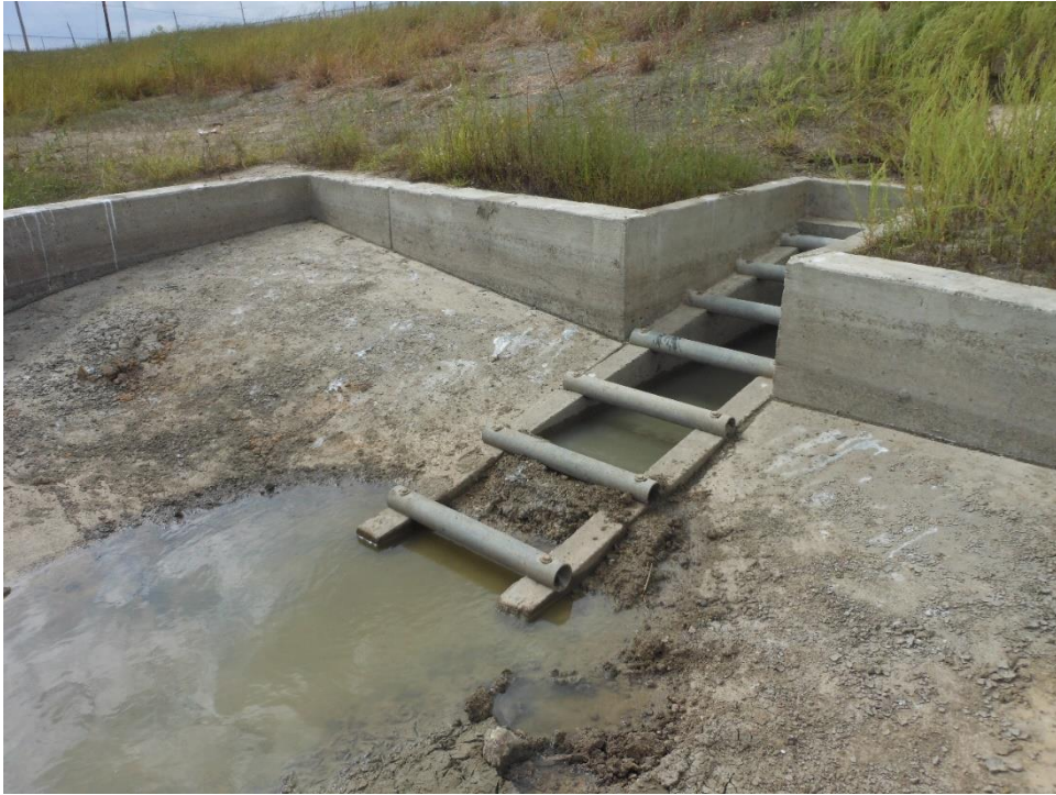
Figure 7 – View of the inside of the control structure pool. Water flows through the screen and into a 24” restrictor pipe.
