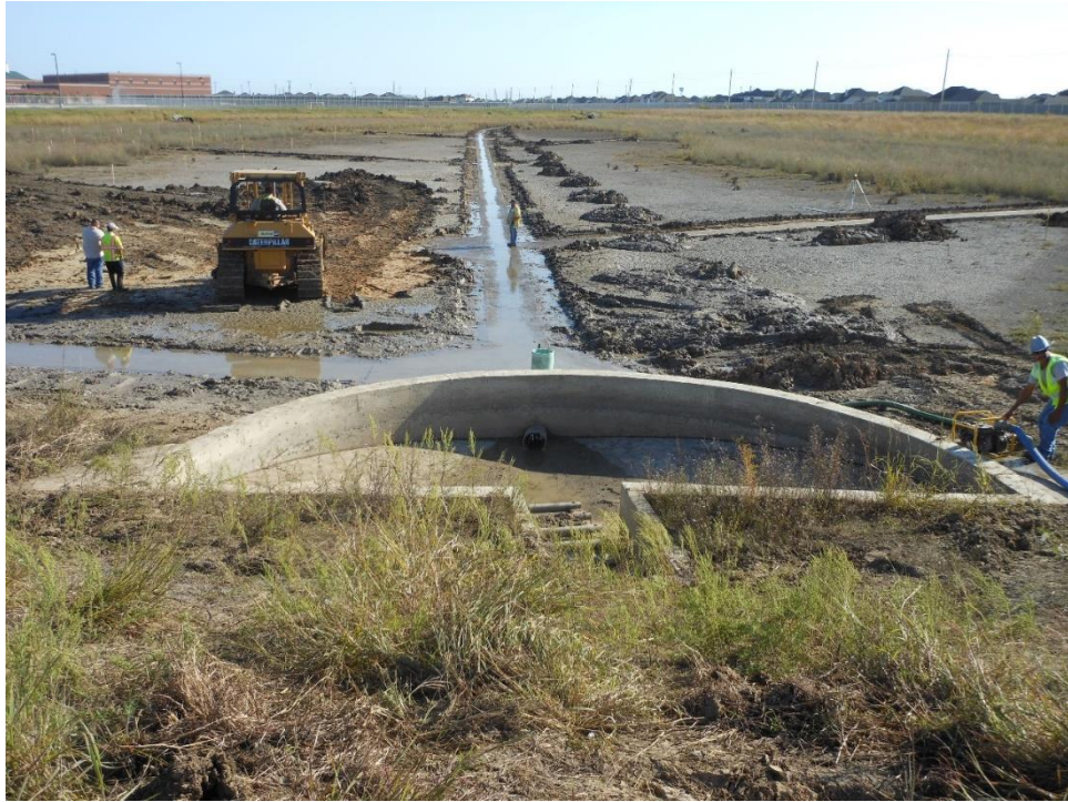
Figure 8 – Retrofitting the detention pond to a wetland involved regrading to allow for plant growth.
