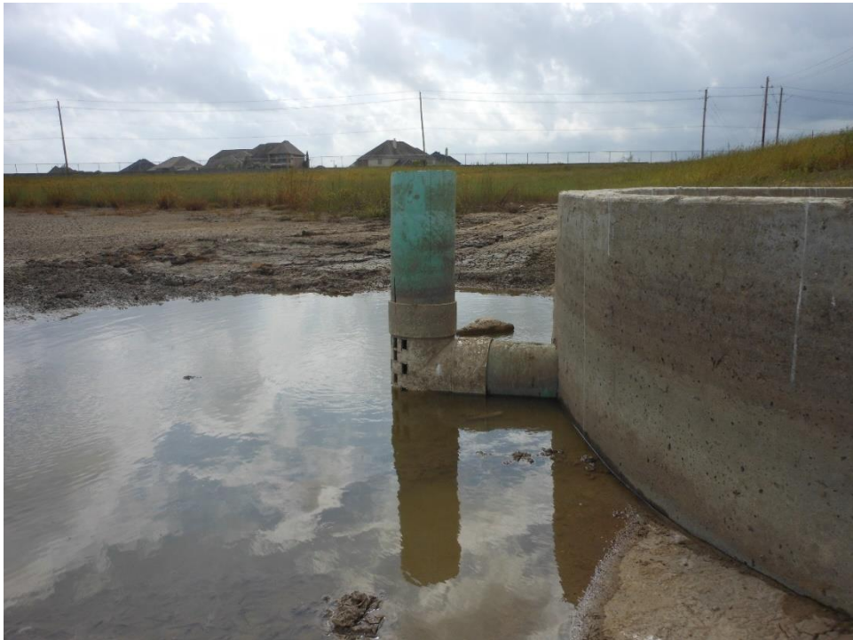
Figure 6 – The friction losses through the 12” inlet pipe and trash screen are the limiting factor for small events. The water level is not normally this low. This picture was taken during the wetland retrofit.
