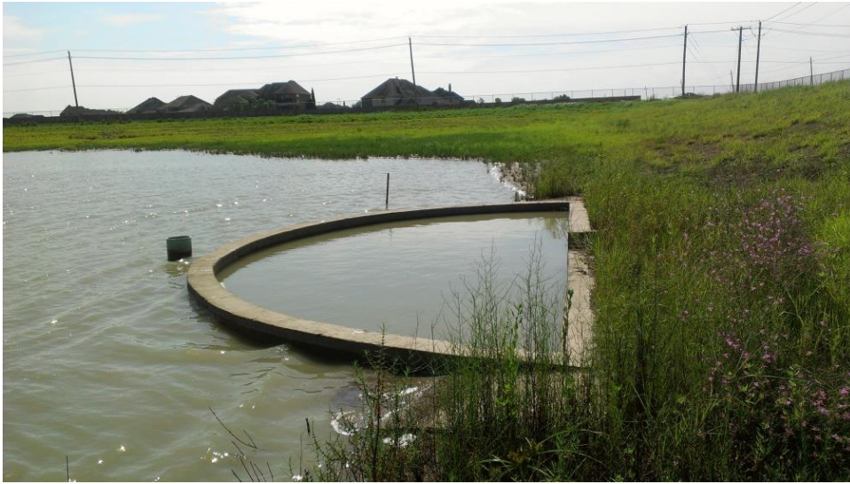
Figure 5 – The outlet control structure consists of a semicircular concrete weir and appurtenances designed to release water slowly
