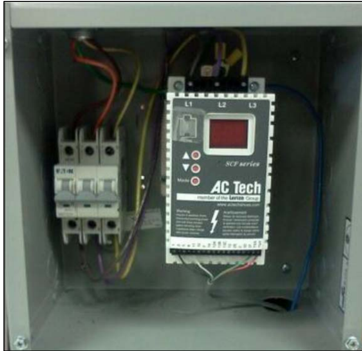
Figure 3-5: The SF430V Variable Frequency Drive mounted in an electrical enclosure box [1]
