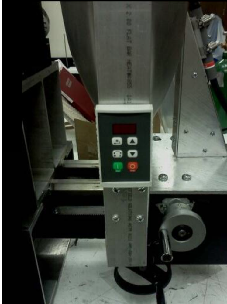
Figure 3-7: Variable frequency drive remote key pad [1]
