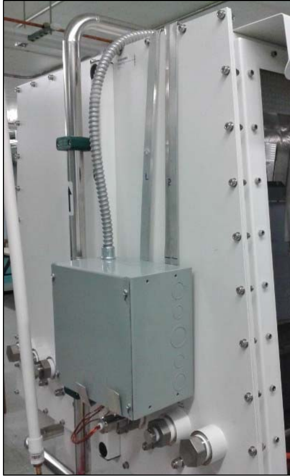
Figure 3-24: Hanging support for the variable frequency drive
