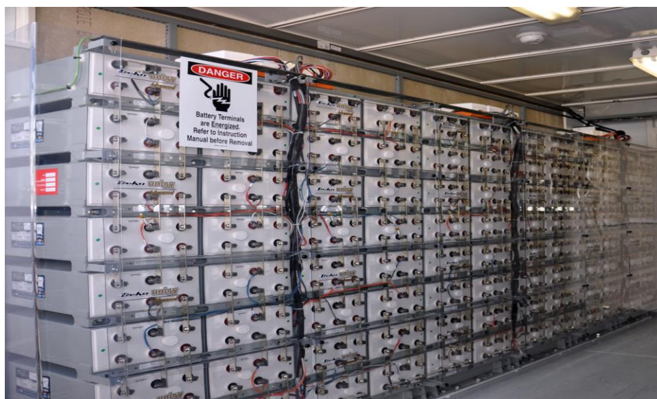
Figure 1.1 Advanced lead-acid batteries energy storage [4].
