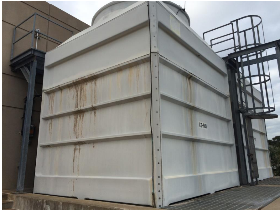
Figure 3.4 Test Facility Cooling Tower
