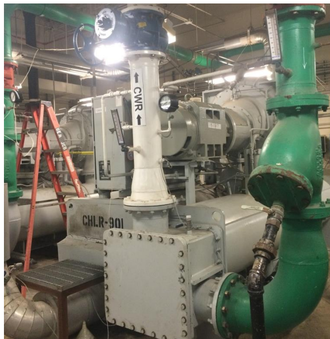
Figure 4.2 A View of the Chiller System
