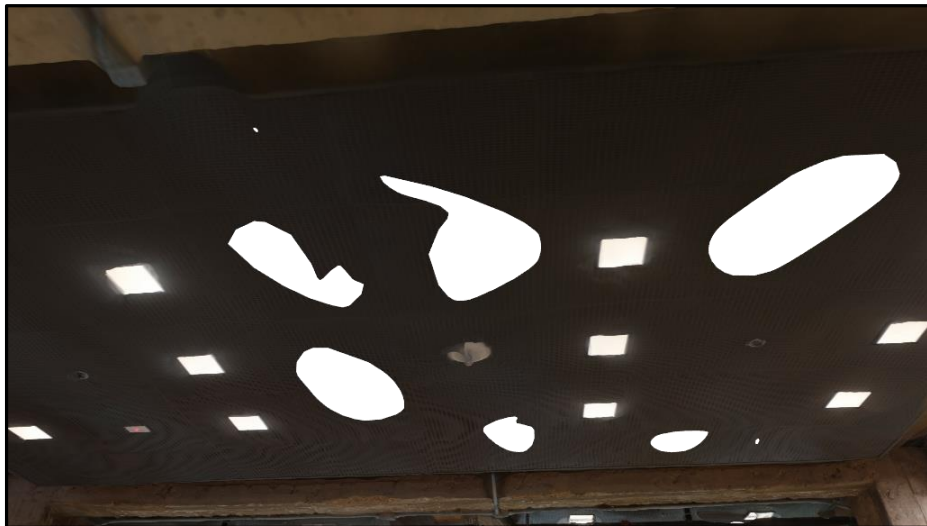
Figure 5.8: Holes appear on repetitive texture pattern ceilings on entry gallery
