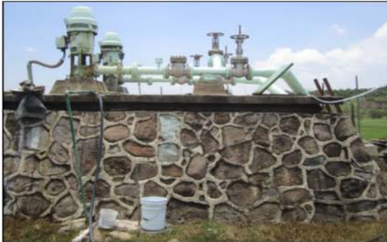
A. Agua caliente pump station and chlorination site part a.
