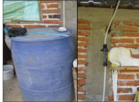
B. Agua caliente pump station and chlorination site part b.
