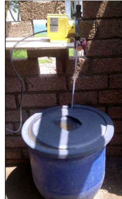
C. Jarrero well chlorination system part a.
