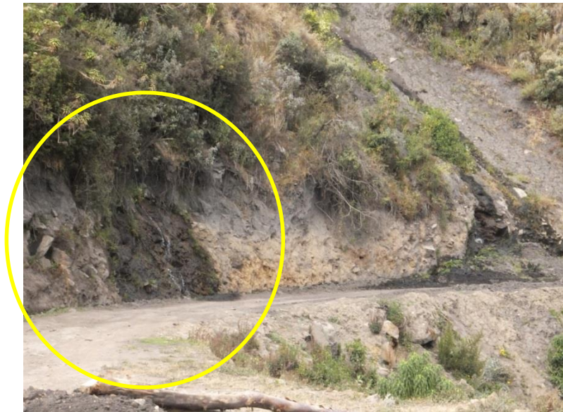
Figure 5.2 A spring flowing into a ditch near the road into Quinchucajas (August 2013)
