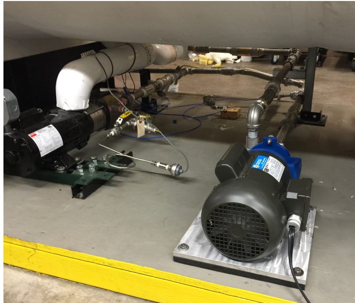
Figure 3.4: The Dayton multistage pump and the Liquidflo 620 centrifugal pump. The suction and discharge piping is shown prior to the placement of insulation.
