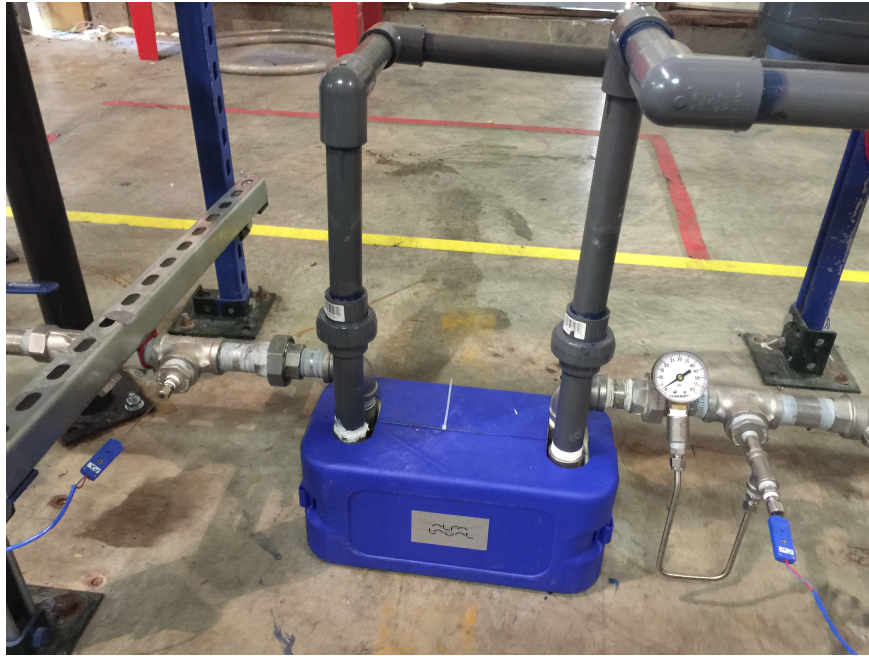
Figure 3.6: The AlfaNova 27-30H heat exchanger shown installed with protective blue thermal insulation. The hot side inlet is shown on the left while the hot side discharge to the pump suction is on the right. The cold side domestic water is shown in 1 inch PVC piping.
