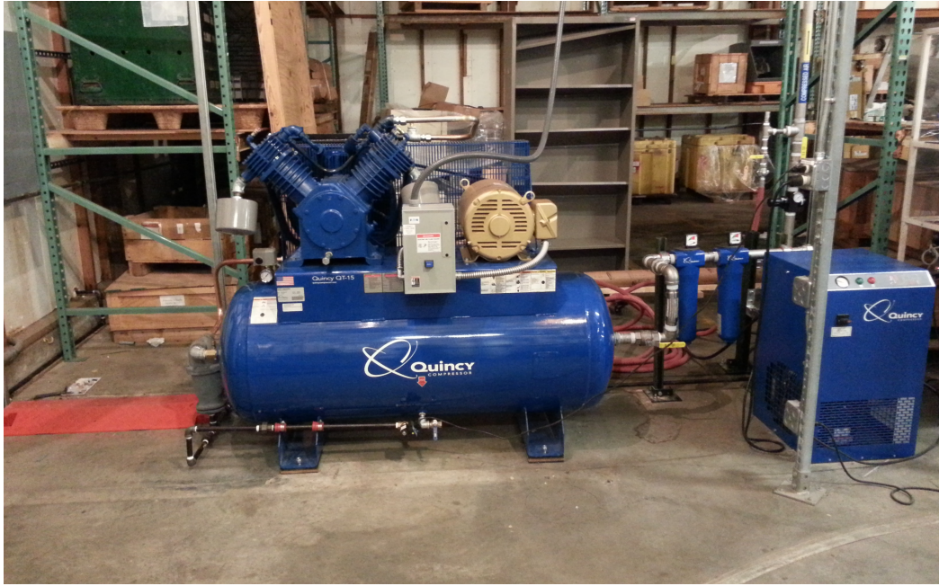
Figure 3.7: The air supply and supporting equipment.
