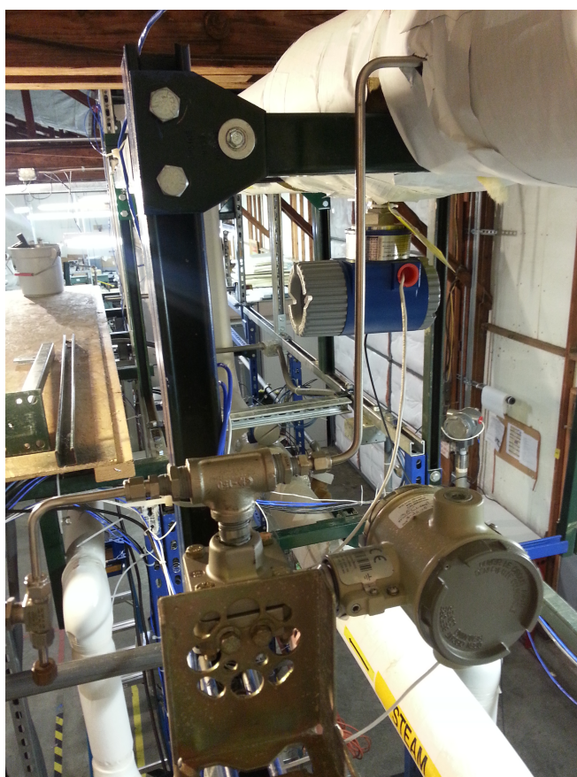
Figure 3.11: The gas outlet absolute pressure transmitter with impulse piping. The transmitter is shown in the foreground while the outlet vortex flow meter is shown in the background.
