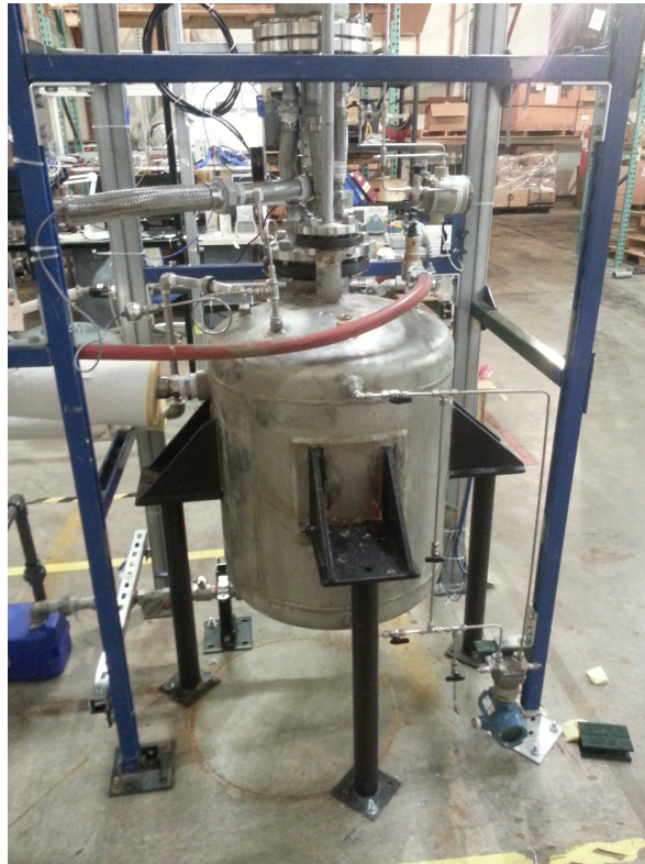
Figure 3.5: The holdup tank shown below the test section before insulation was applied. The two inch coupling and piping shown on the left side were later removed and plugged after this photo was taken.
