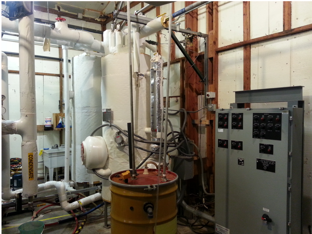
Figure 3.9: The steam generator shown with insulation. The control panel is on the right and the blowdown drum is shown in yellow.
