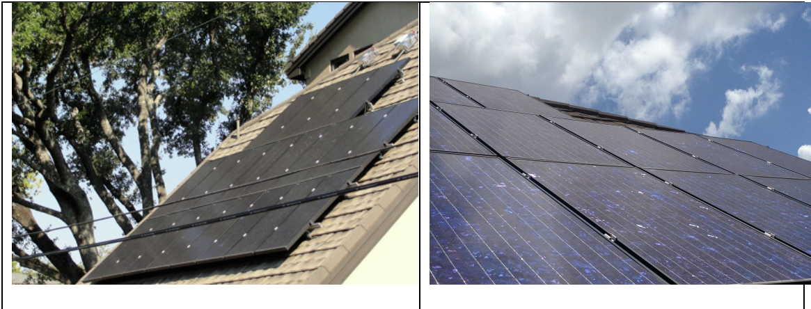
Figure 18. Street (left) and close-up (right) views of the solar photovoltaic system (SPVS)
