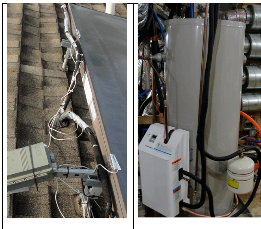
Figure 21. Solar thermal collector, heating appliance and hot water storage tank
