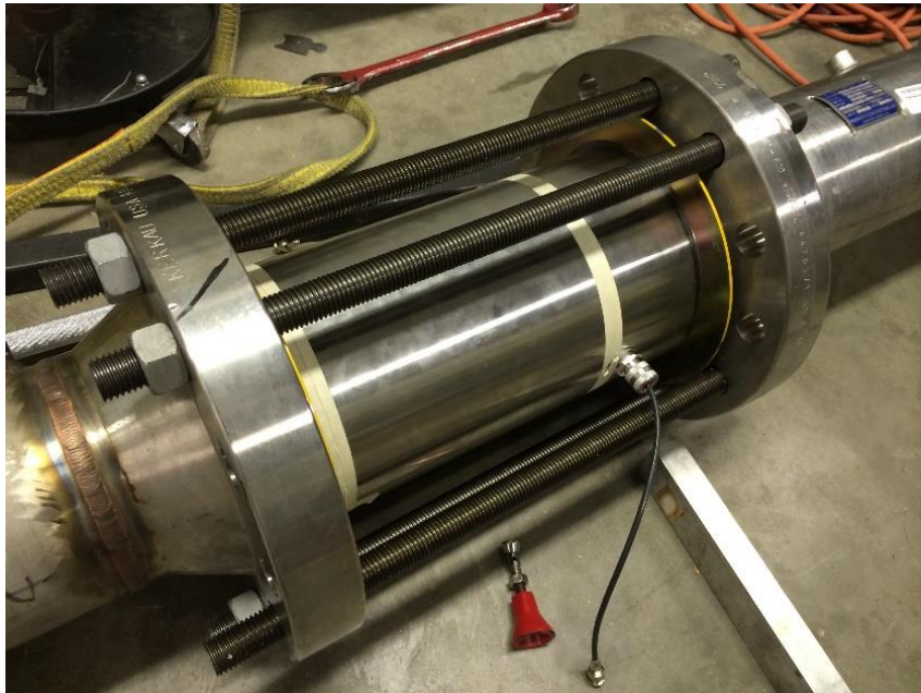
Figure 35. MPFM being installed between two pipe flanges. Electrical connections installed on sides.
