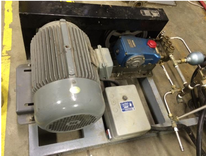
Figure 27. Seal flush pump skid (disconnected during disassembly)
