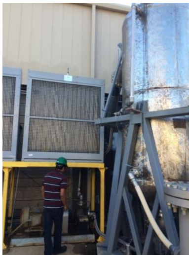
Figure 28. Heat exchanger fan and pump (left) and large stainless steel tank for water/air reservoir (right).
