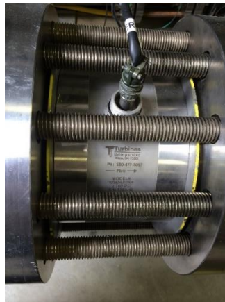
Figure 22. Turbine meter used to measure water flow in the inlet line
