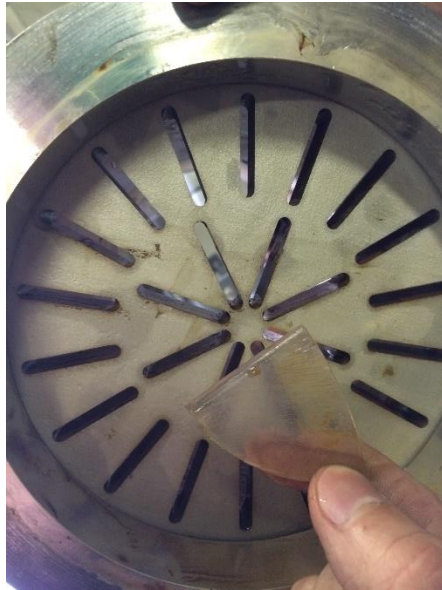
Figure 50. One of the plastic pieces found before the slotted plate during disassembly
