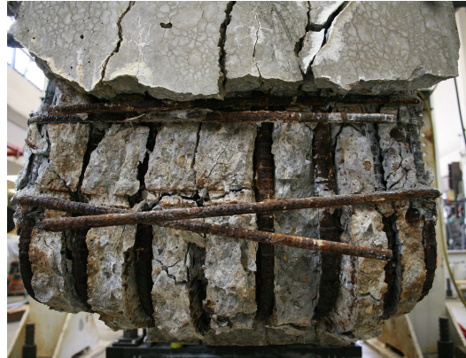
(d) Anchorage Debonding of U-bars, and Lateral Displacement of Longitudinal Steel, in the External Beam-Column Joint
