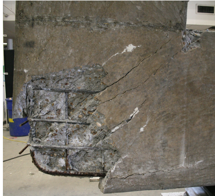
(c) Interior and Exterior Corner after Removal of Spalled Concrete (Opposite Face Shown in b)
