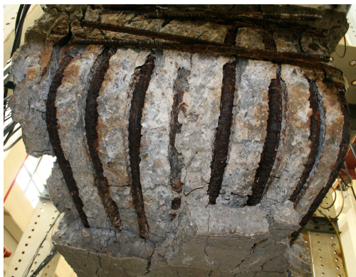
(e) Under Side of Exterior Corner Joint after Removal of Spalled Concrete
