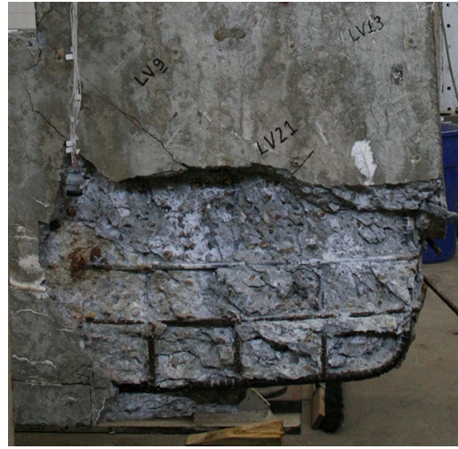
(b) Exterior Corner after Removal of Spalled Concrete (Opposite Face in c)
