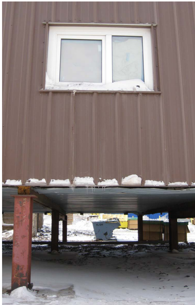
Figure 46: The wall and ground floor connection showing some ice problems.
