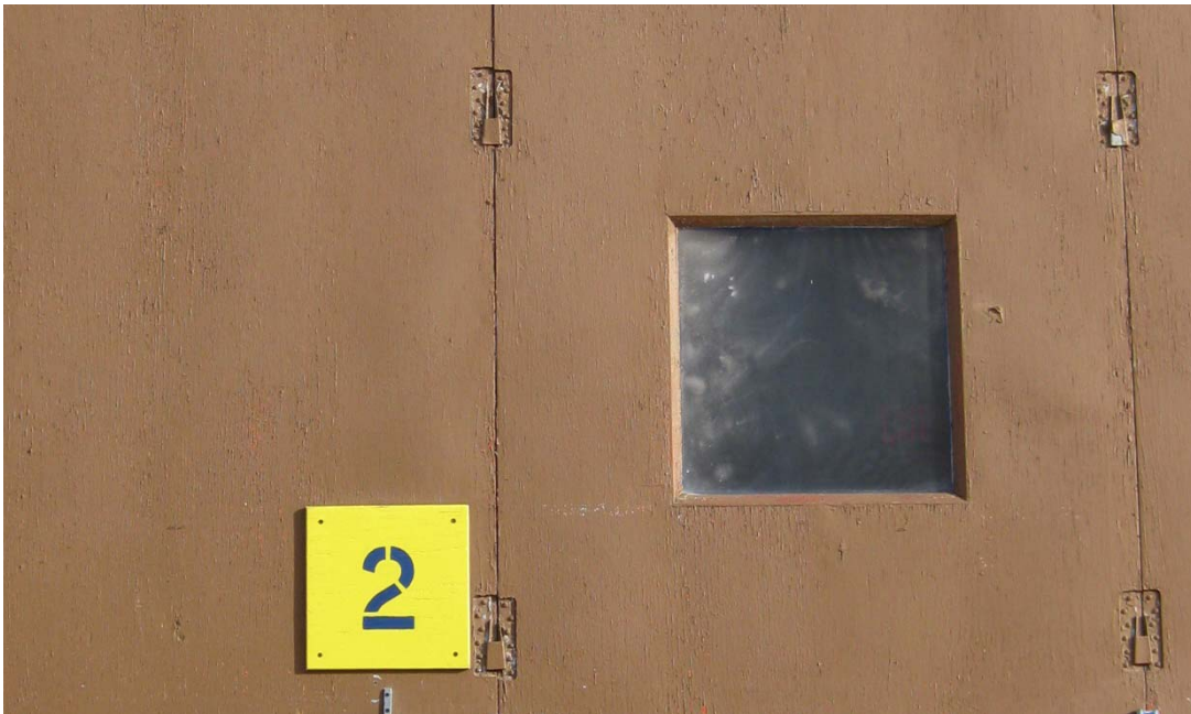
Figure A- 27: Detail of the exterior wall of the “Gerbil Gym” showing four clip fasteners and a window. Photo by author, 2009.
