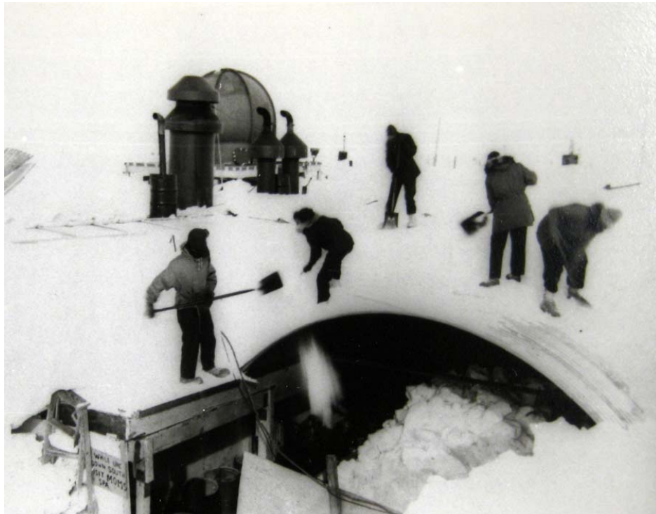
Figure A- 33: Men removing snow from the entrance to South Pole Station, Antarctica, to ease the strain on the supporting timbers to that they may be rebuilt. Operation Deep Freeze '65. Photo by PH3 Jerry W. Lakso. Courtesy U.S. National Archives, College Park, MD.
