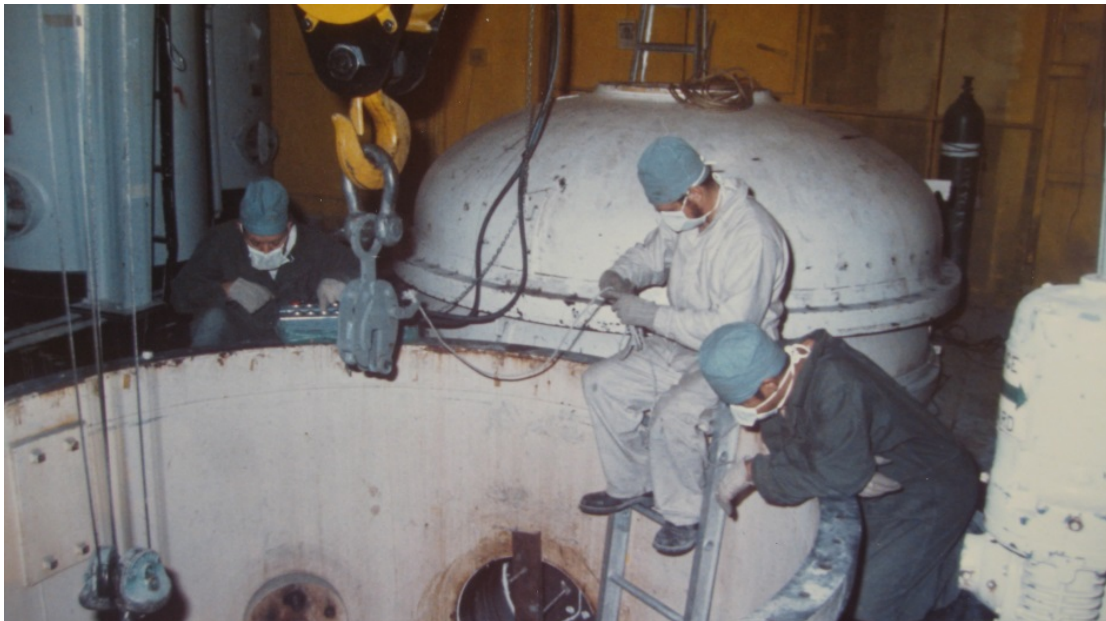
Figure A- 67: A view of a shield replacement at the nuclear power plant. McMurdo Station, Antarctica. November 19, 1974.
