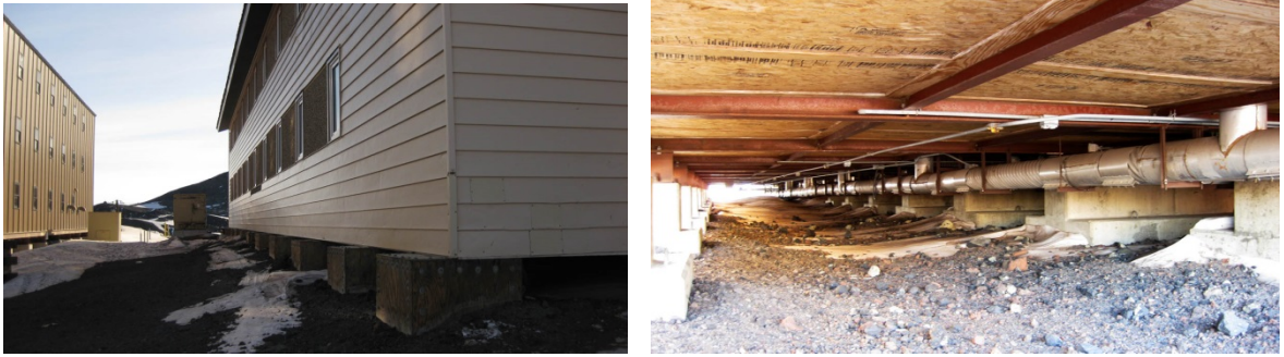
Figure 47: Dorm 203 with its low foundation (left) and a view of the underside of the building, showing its cladding, piping, and low clearance.
