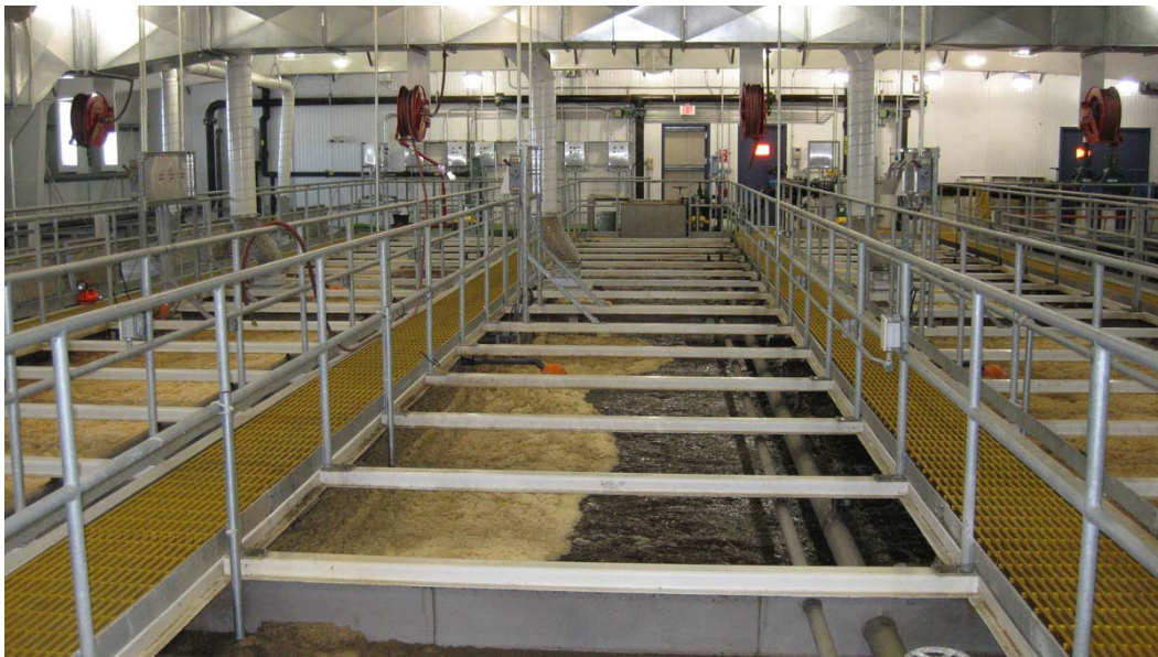
Figure A- 73: Inside McMurdo's wastewater treatment facility
