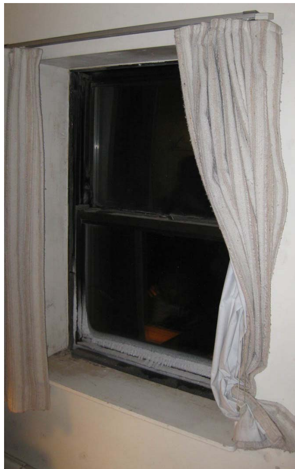
Figure A- 61: Window with curtain, showing moisture, spindrift, and icing problems. Photo by author, 2010.
