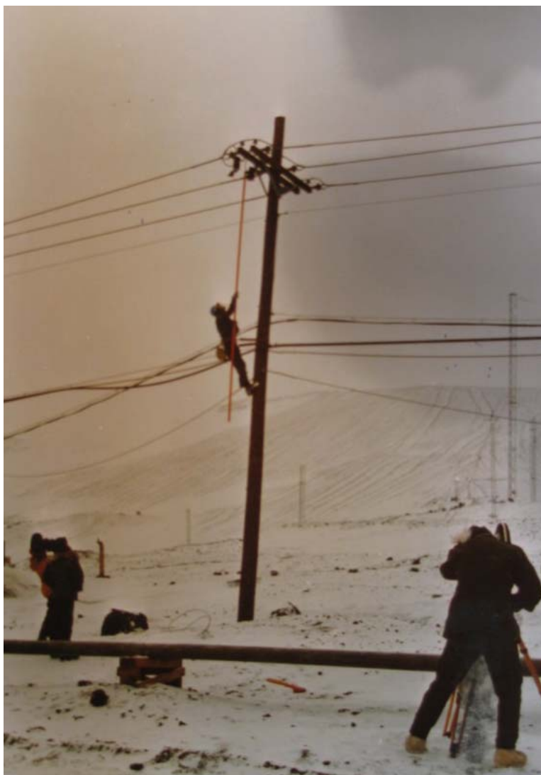
Figure A- 52: Photographer's mate First Class Robert L. Zeisler, left background, and Photographer's mate Third Class Alan T. Brown, right, film activity as a lineman repairs a utility pole. Naval Photographic Center, Naval District, Washington, D.C. Official Nvy photograph. November 13, 1987. Photographer: Charles J. Williamson. Courtesy U.S. National Archives, College Park, MD.
