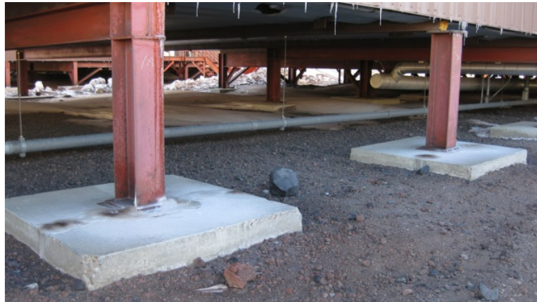
Figure A- 58: Example of a concrete footing in McMurdo Station. Photo by author, 2009.
