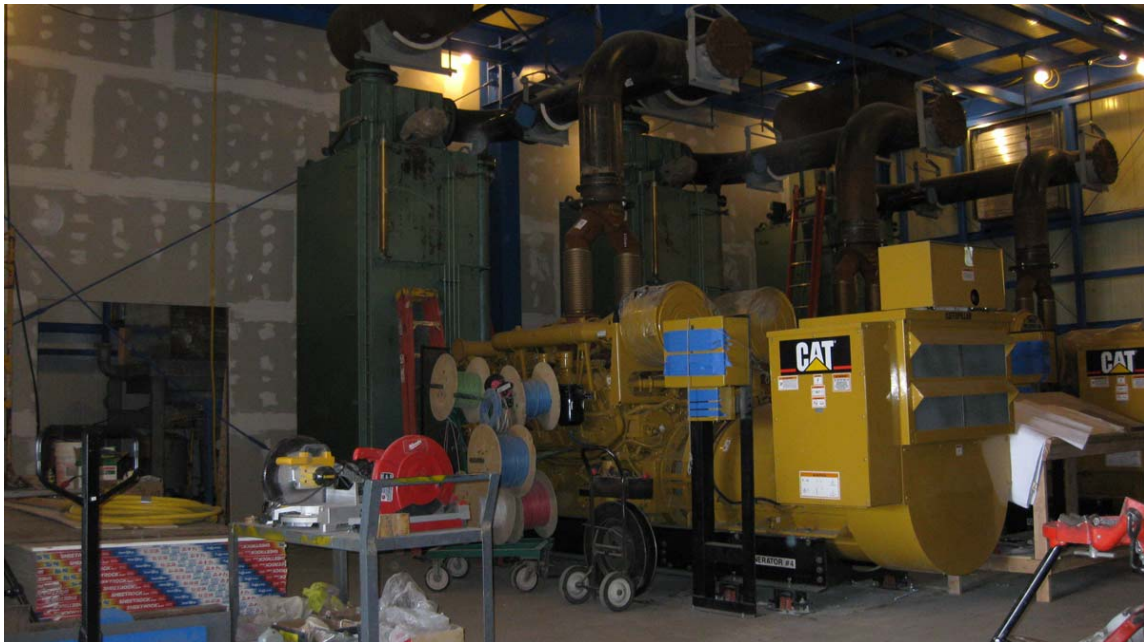
Figure 32: Generators in their new housing facilities in McMurdo Station, 2009. Photo by author, 2009.
