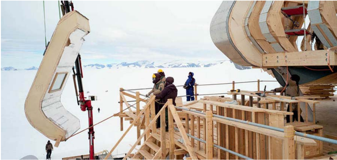
Figure A- 46: The thick layers in the walls reportedly allow the station to be completely passively heated Project © International Polar Foundation. Engineering and Technical Design for the Structure and the Shell © Philippe SAMYN and PARTNERS.
