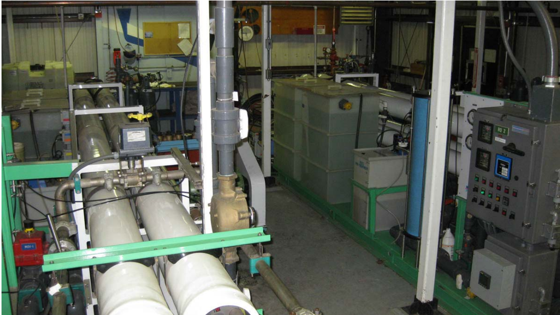
Figure A- 72: Just some of the equipment used in the RO process in McMurdo's water treatment facility.
