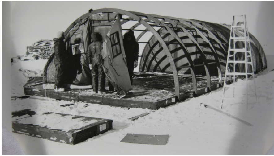
Figure A- 21: Byrd Surface Camp, Antarctica. Jamesway tent under construction during the Deep Freeze 1980 season. (Note the flooring.) Photographer: Jeff Hilton. Date: Nov. 6, 1979. Naval Photographic Center, Naval District, Washington, D.C. Official U.S. Navy Photograph.
