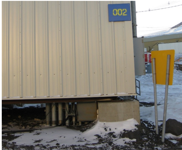
Figure A- 60: Example of a concrete footing in McMurdo Station. Photo by author, 2009
