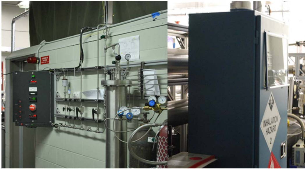
Figure 5. Left: gaseous manifold, against blast wall to test cell. Right: CO safety cabinet; CO ran from cabinet into the manifold connecting at the circular valve (center one of the five visible in picture).
