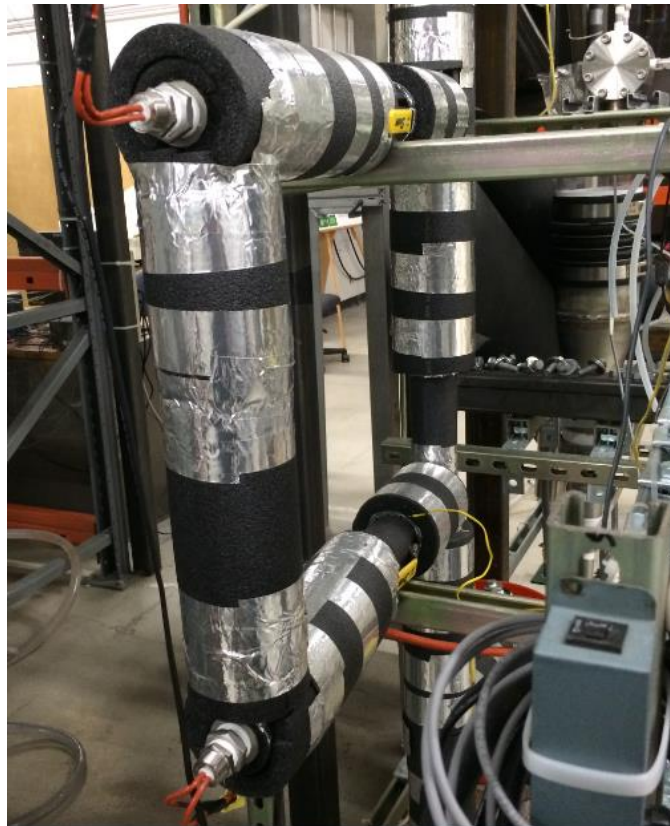
Figure II.3. 7. Heating loop (7kw)
