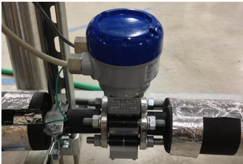
Figure II.2. 6. Magnetic flow meter
