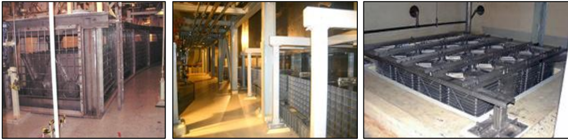
Figure I. 2. Containment sump strainers
