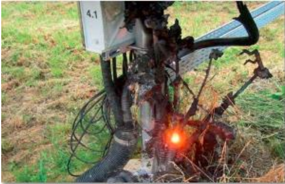
Figure 3.4: Glowing arc in the DC wiring near a combiner box [72]
