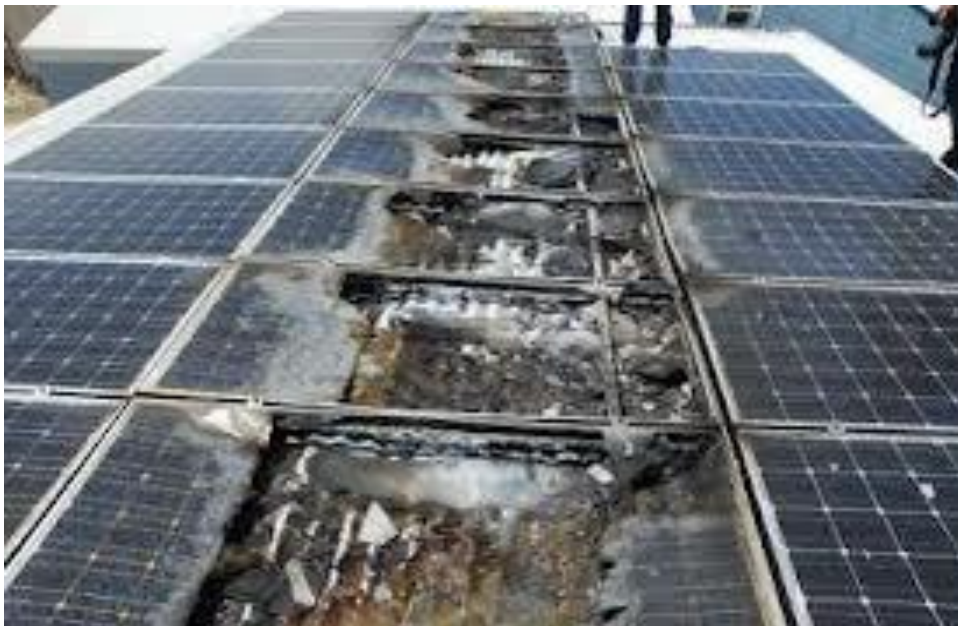
Figure 3.5: Fire damage to a roof-mounted PV array [73]
