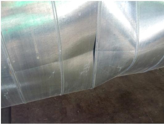
(a) Seam Failure
