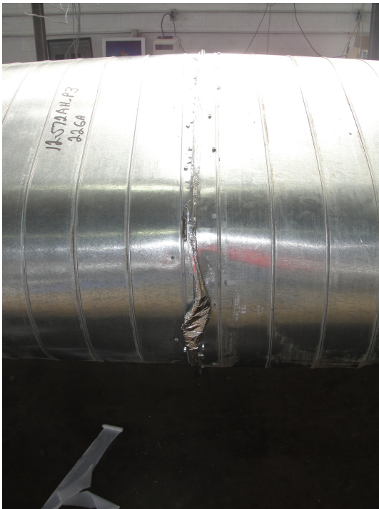
(c) T-25 Failure
