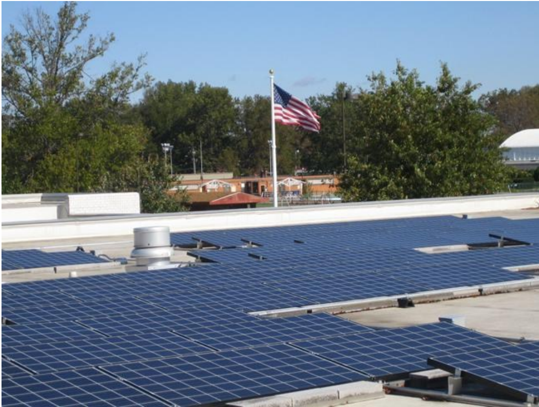
Figure 6.3: Solar panels atop a library roof in Euclid, Ohio
