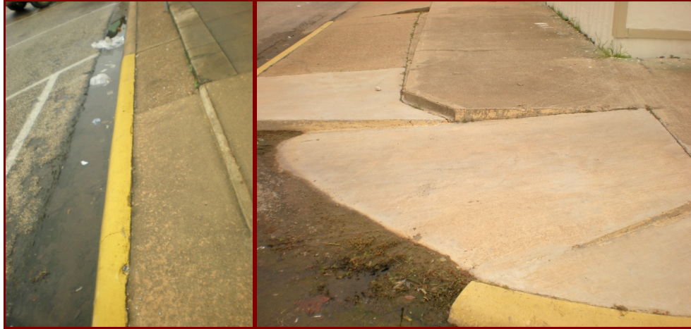
Figure 1.6 Drainage along sidewalks in Sealy
