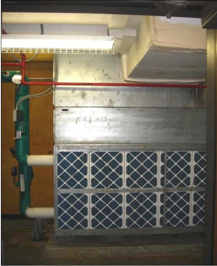
Figure 206: Air Handling Unit in the 5th Floor of the John Connally Building
