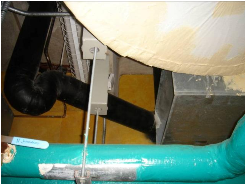
Figure 207: Installation of a Portable Logger to Measure the Return Air Temperature of an AHU on the 5th Floor
