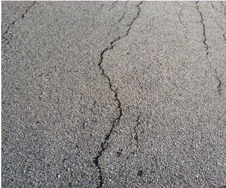
Figure 6. Low temperature cracking
