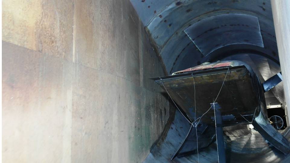
Fig. 8: View of downwind side of motor housing, showing the large diffuser angle off of the housing and the wood inserts on the tunnel walls.
