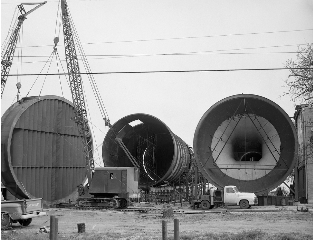
Fig. 6: The 30 ft diameter turning vane section of turn three can be seen here during the construction of the tunnel shell in 1958 [4].
