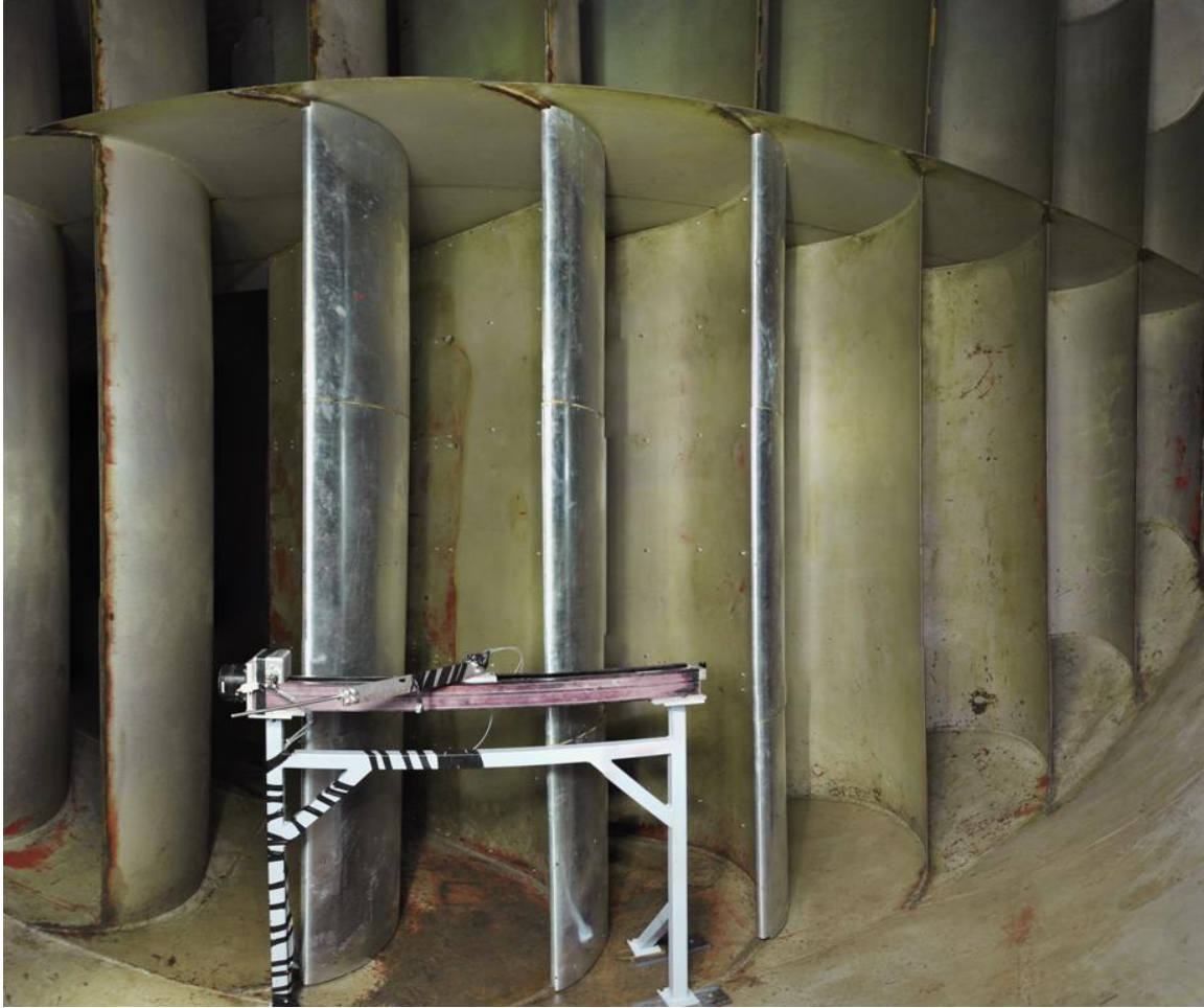
Fig. 30: Upwind view of turning vane proof of concept modifications in place with traverse mechanism.
