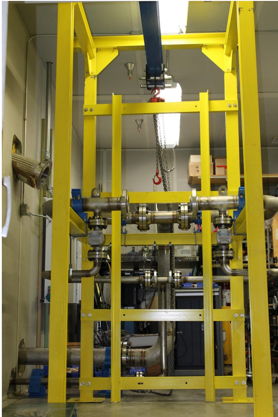
Figure 35 Pump rig support structure with monorail crane
