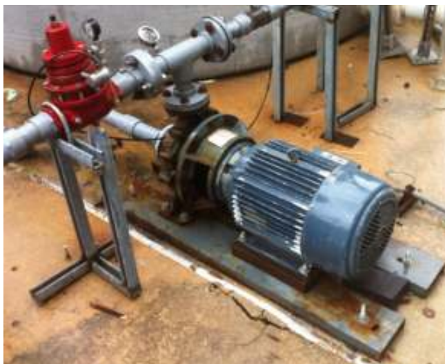
Figure 5.2 Centrifugal Pump And Pressure Regulator.
