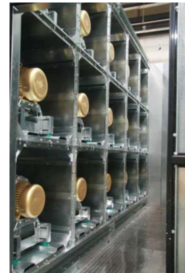
Fanwall AHU (TRIP)
