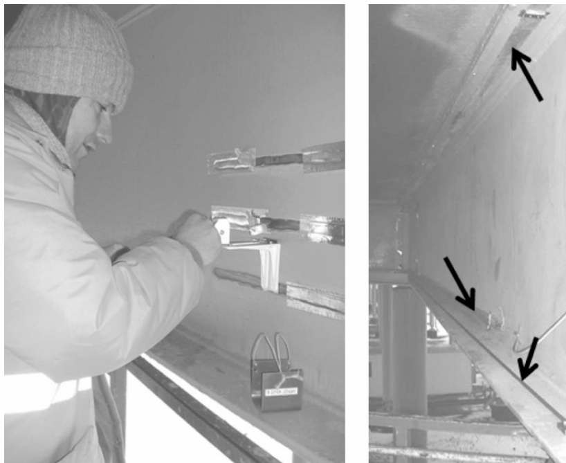
Figure 5-6. Installation of Distributed Sensors (left) and Installed Distributed Sensors (right) (Glisic and Inaudi 2010).
