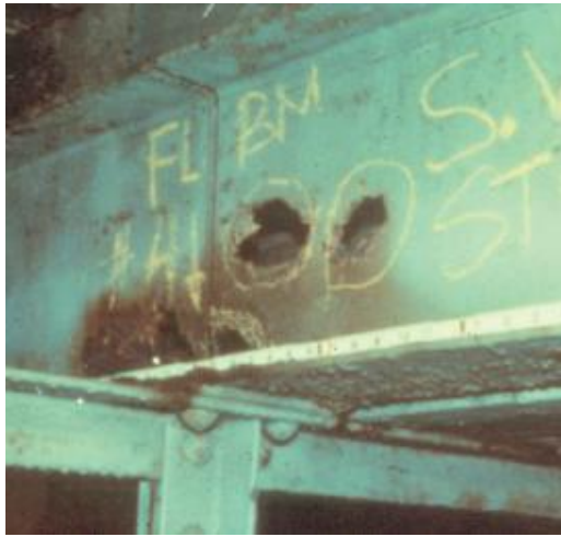
a) Corrosion (Ryan et al. 2006)
