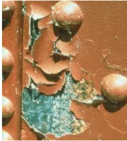
b) Paint Failure (Ryan et al. 2006)
