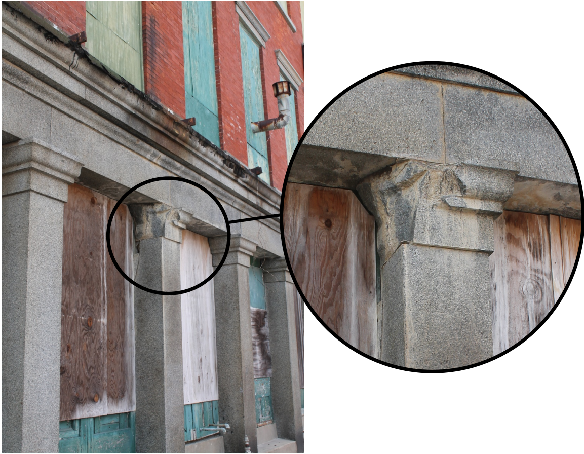
Figure 2.10. Hendley Building, showing damage caused by a shell from USS Owasco . Photograph by Jessica R. Stika.
