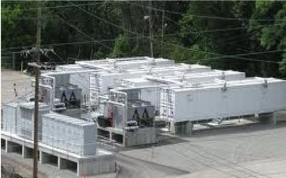
Figure 36. Example of Battery Complex in Northern Chile
